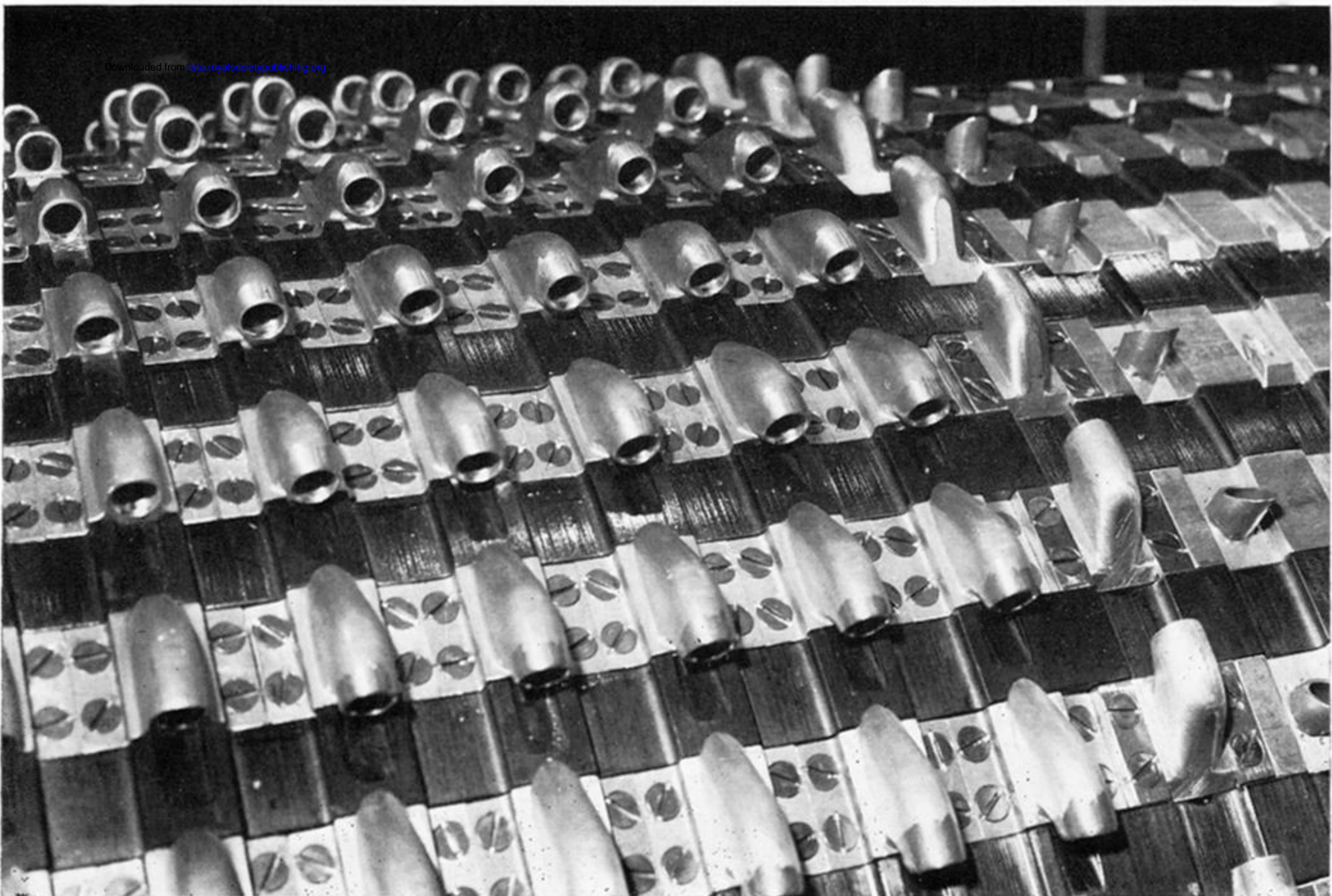
FIGURE 7. Generator stator core with segregating baffles.
